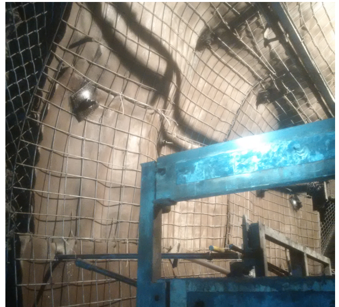
CC attached to galvanized screens for support
