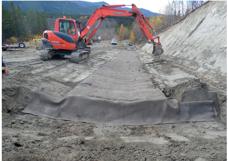
CC edges were captured in a large anchor trench which was later backfilled
