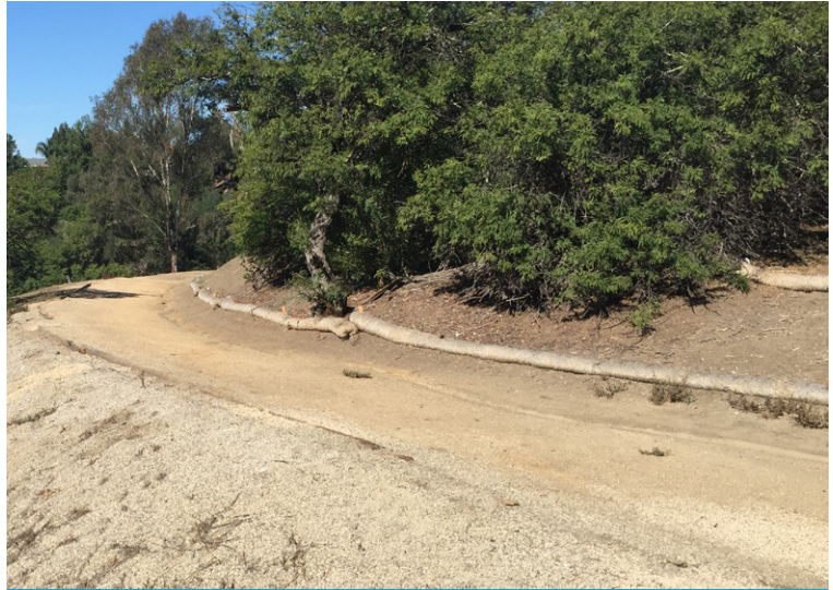
Existing drainage system
